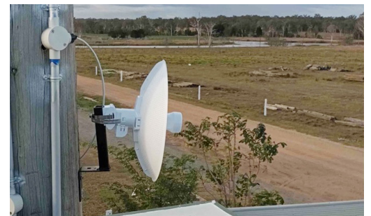
➤ D-Link Long Range Wireless Bridges implemented to deliver long-distance Wireless Connectivity between farm buildings
