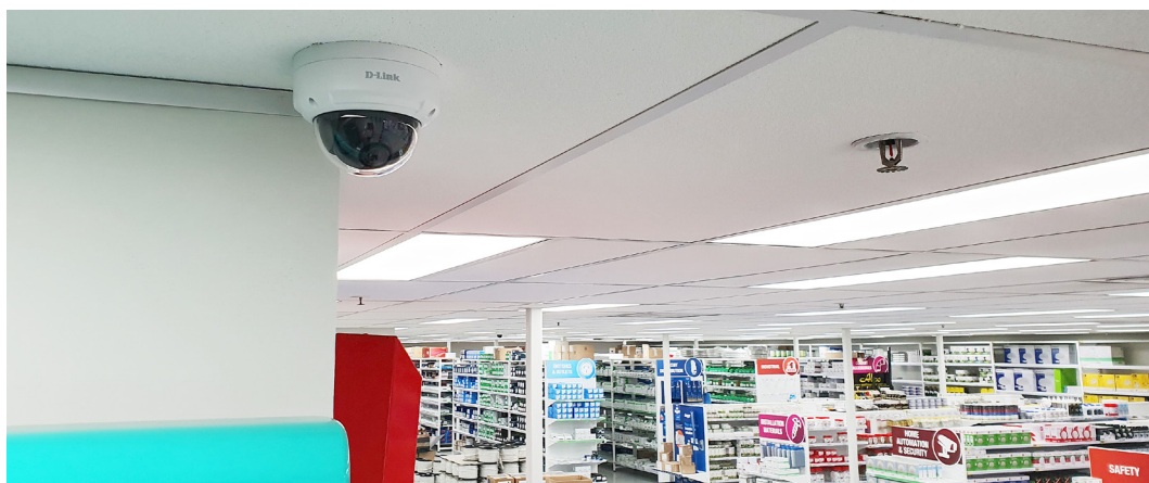
Photo above shows D-Link IP Cameras in use and in-situ at Lawrence & Hanson's brand-new showroom in Brisbane.
